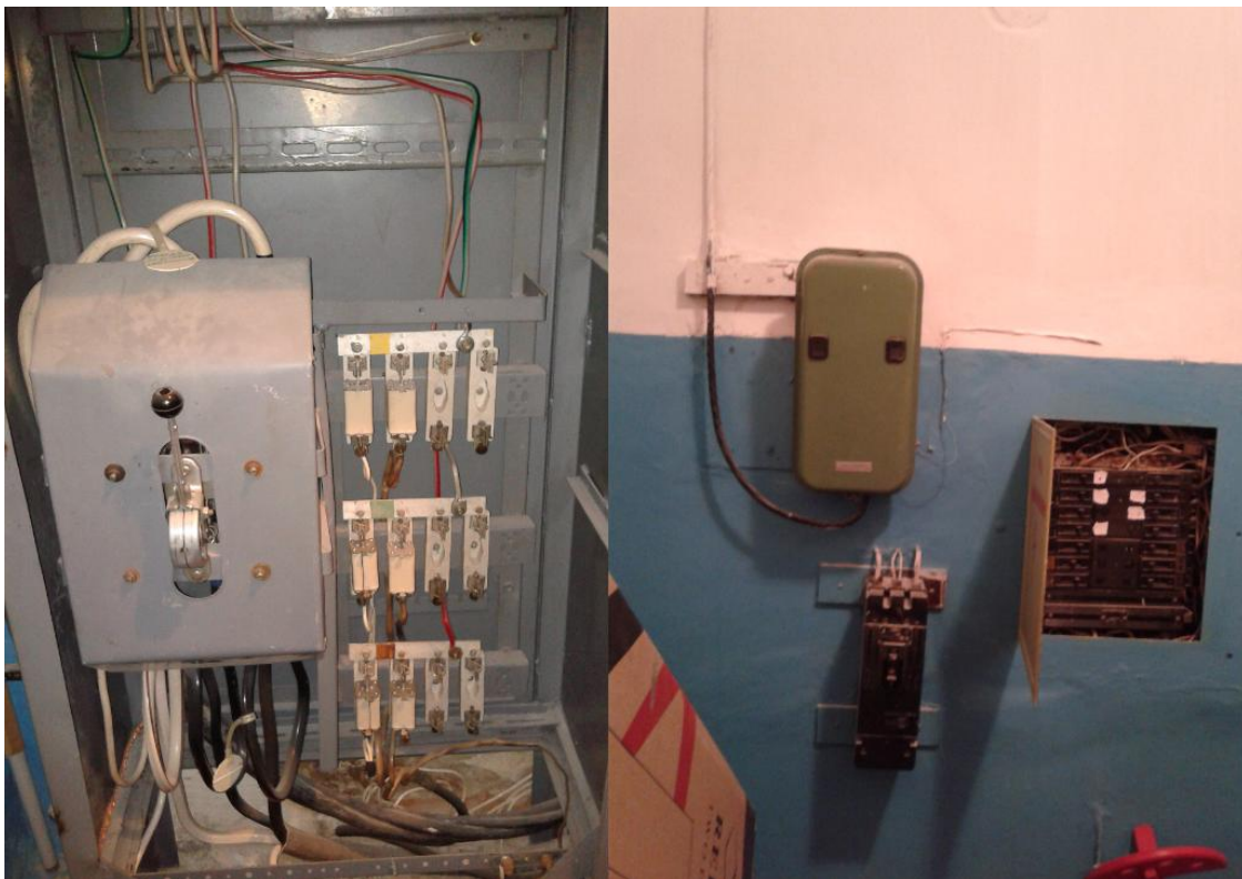
15. figure: Electric equipments and fuse box
