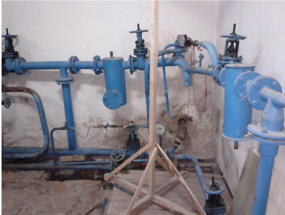
13. figure: District heating pipes in the mechanical room
