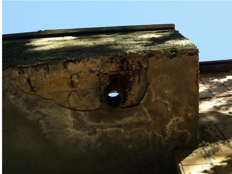
12. figure: Corroded drainage opening
