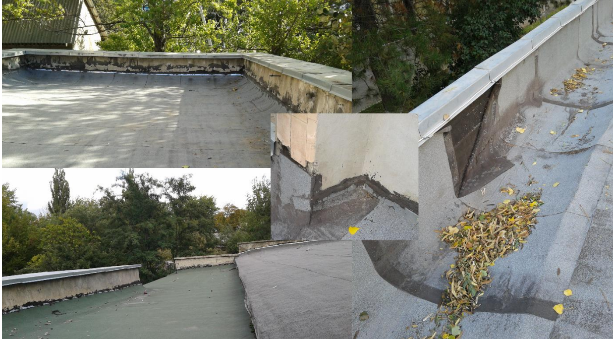
11. figure: Image compilation about the condition of the roof
